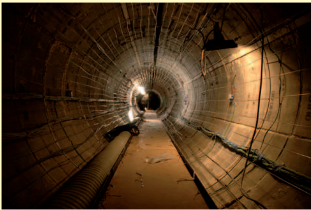
The heating system is fixed to the wall of the PRACLAY gallery.
