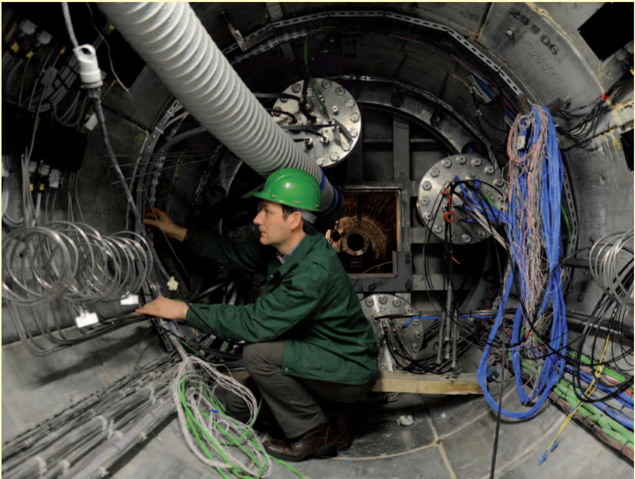
A researcher checks the measuring instruments near the metal structure sealing the gallery.
